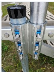
316 SS Square Nuts Installed in Stair Hardware
